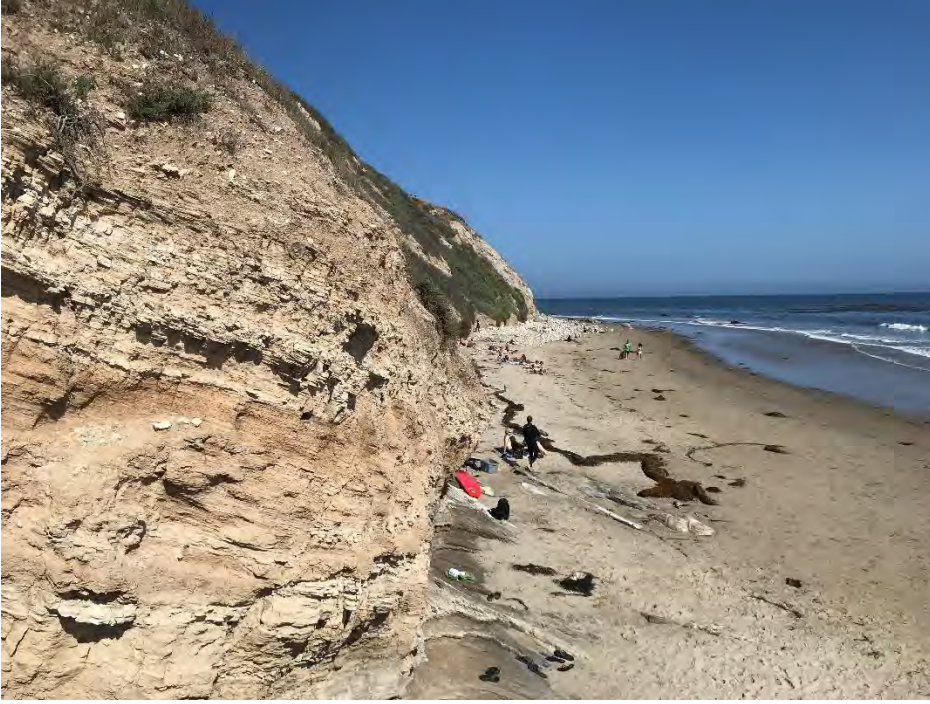
Top of Bluff Showing Daylighted Monterey shale Beds – View to East of from Mesa Lane Staircase (near CoSMoS Transect 4007)
