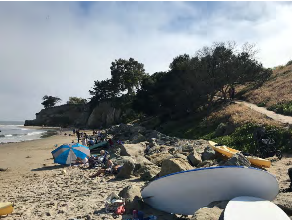
- Revetment and Fill Slope at Leadbetter Beach near Santa Barbara Point; View to Southwest (near CoSMoS Transect 3977)
