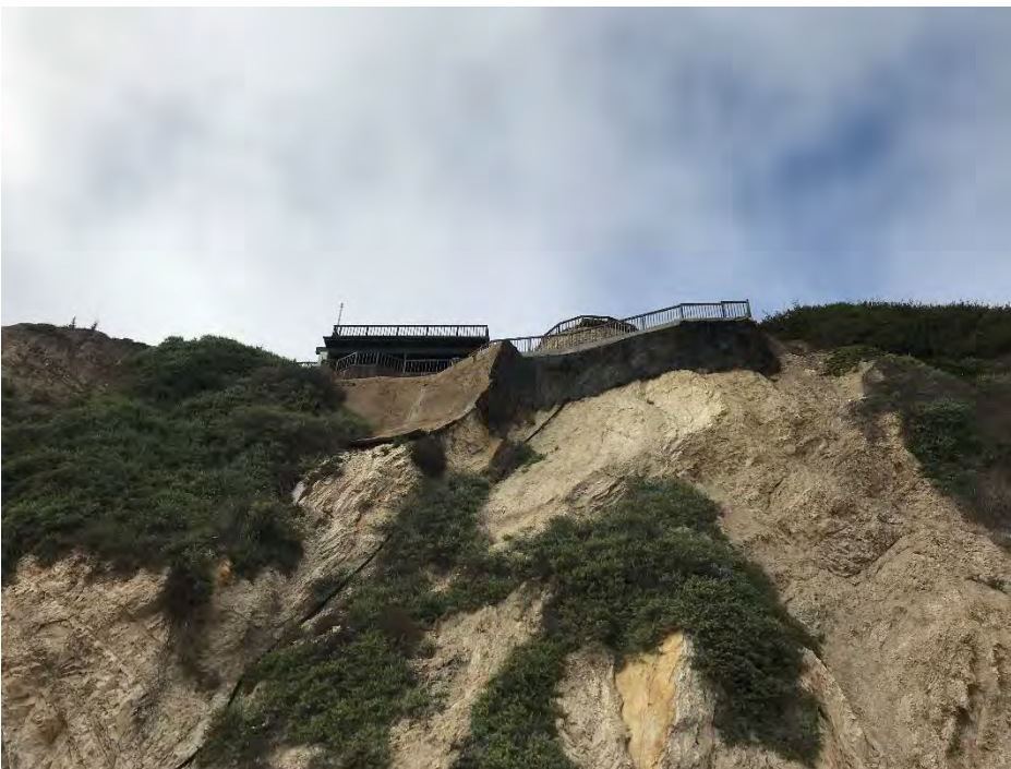
- Seacliff and Residential Structure West of Thousand Steps and East of SB Lighthouse (West of CoSMoS Transect 3992)
