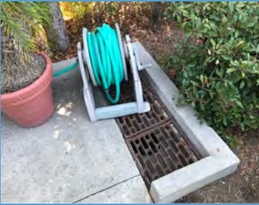
Drainage drop inlet
