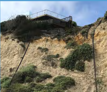
Drain pipes directing water to the toe of the bluff
