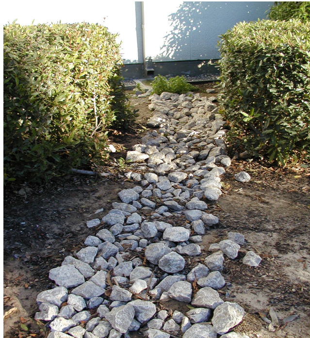
Figure 5-2: Flow Spreading - Directing runoff from a disconnected downspout away from a foundation (University of California, Santa Barbara)
