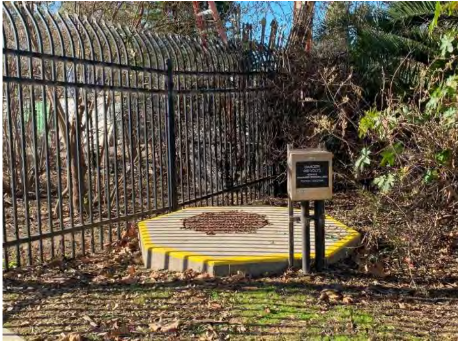
Figure 4-14. Manhole 1B at the El Estero WRC
