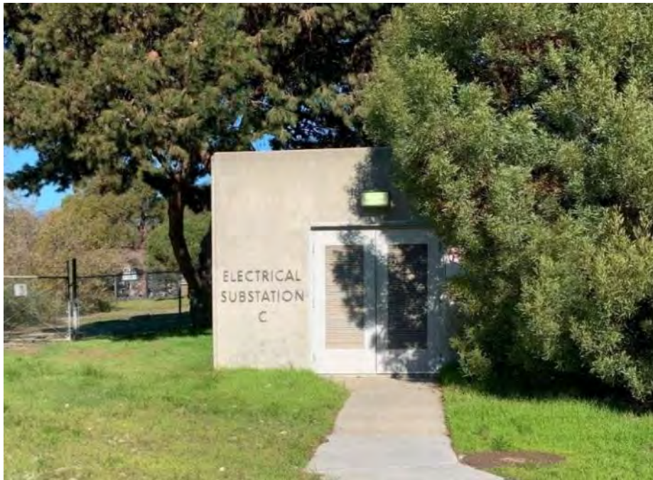
Figure 4-7. Electrical Substation C
