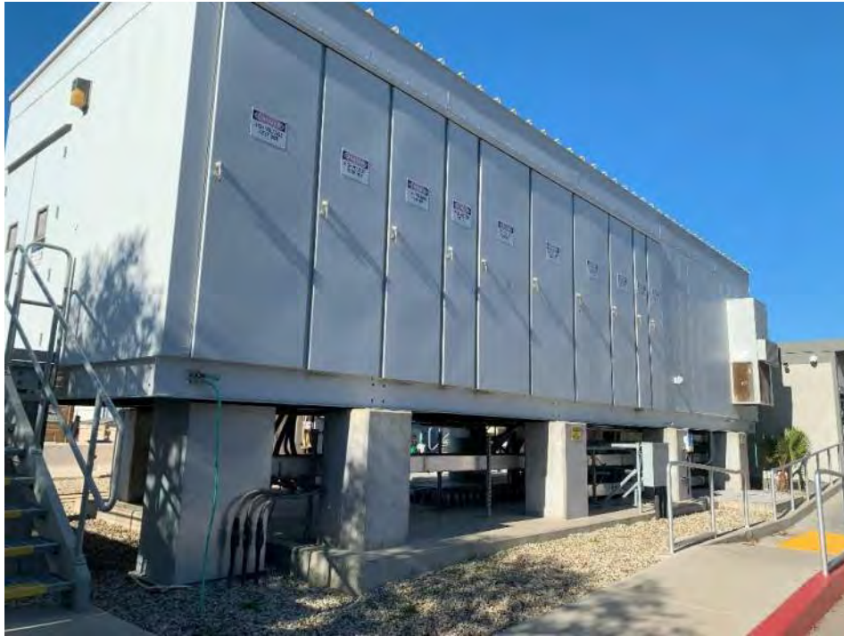
Image Note: Photo of Desalination Plant electrical equipment is 14.2 ft, which is approximately the FEMA base flood elevation plus 1-foot.
