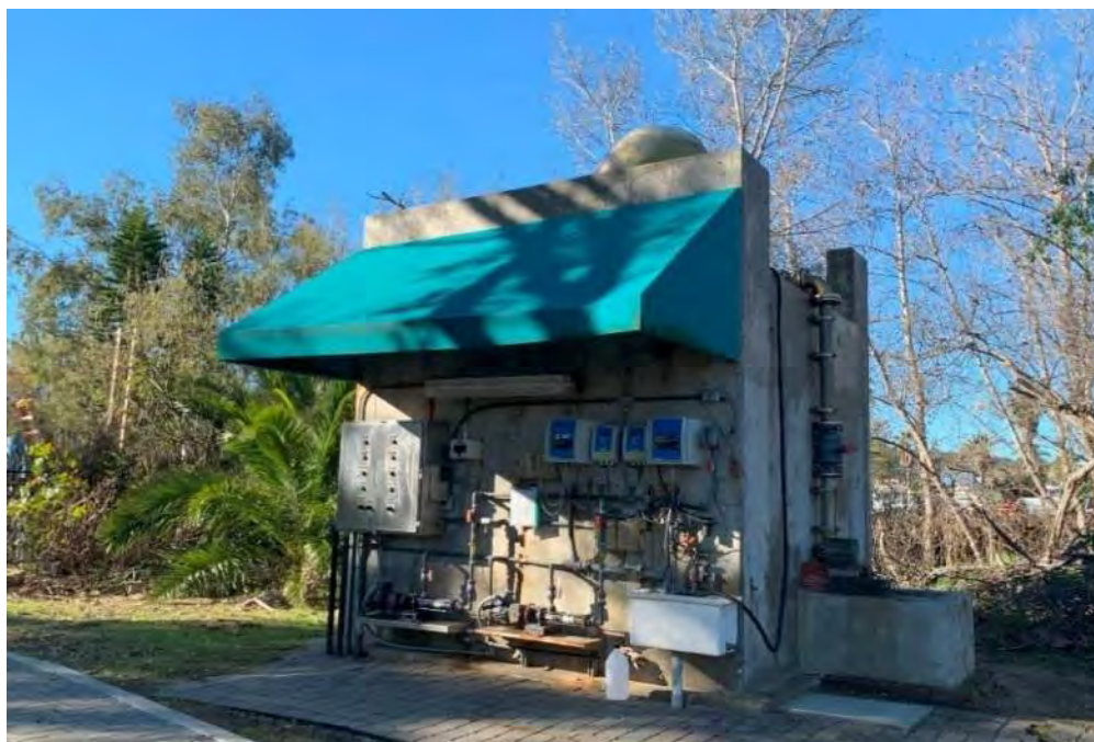
Figure 4-8. Electrical Systems at the Brine Box
