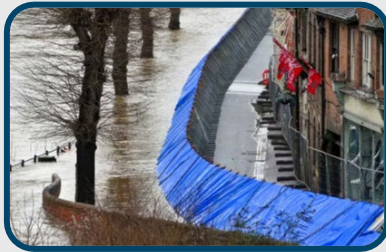
1 Deployable flood proofing
