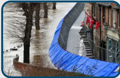
1 Deployable flood proofing
